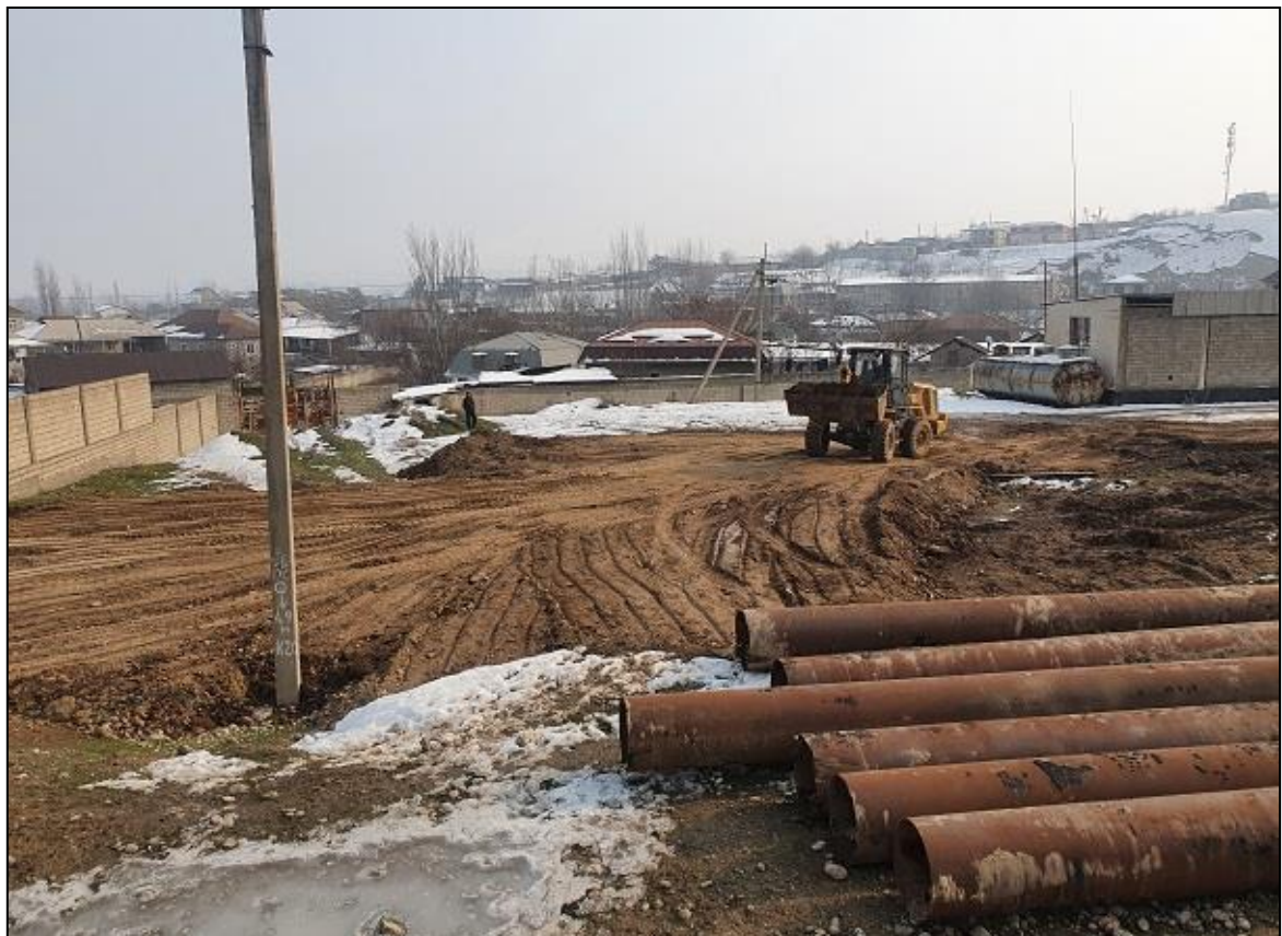
No 2. Photo of further reinstatement (filling) work conducted on the land parcels located at km 7+350 - km 7+645 LHS of Dushanbe -Kurgonteppa Phase 1. All works being carried as requested by the affected persons and agreed by all parties.
