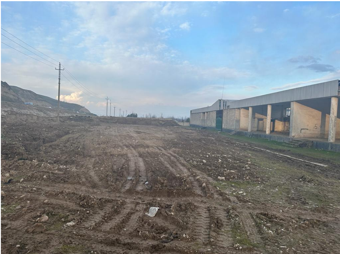
Photo No 4. Contractor followed the request to the owner and gathered some soil on one side of the land parcel to alleviate the level of ground surface
