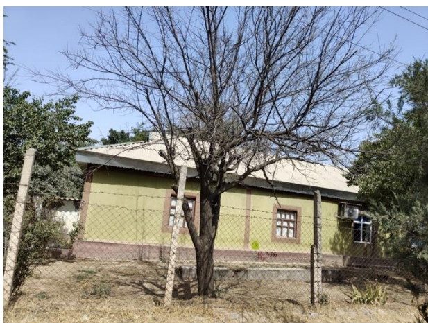
Affected residential structure
