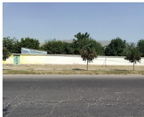
Affected boundary wall of a residential structure
